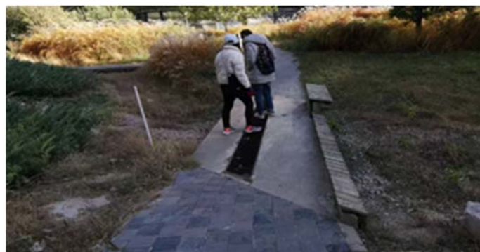
(P5-2: The uneven pavement)
